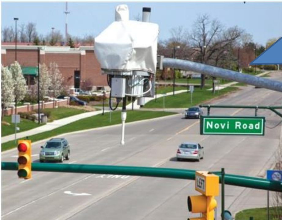
DSRC roadside unit located in Novi, Michigan
